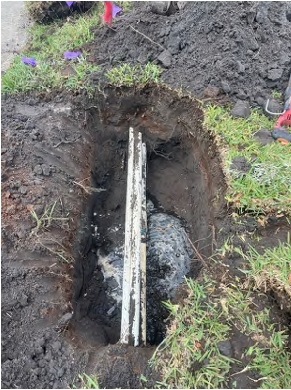
3" mainline leak exposed
